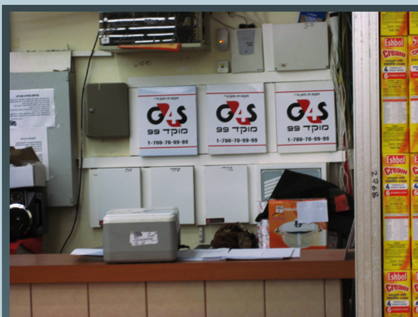
Systems of G4S installed in a supermarket in the West Bank settlement of Modi'in Illit. Photo: DanWatch
